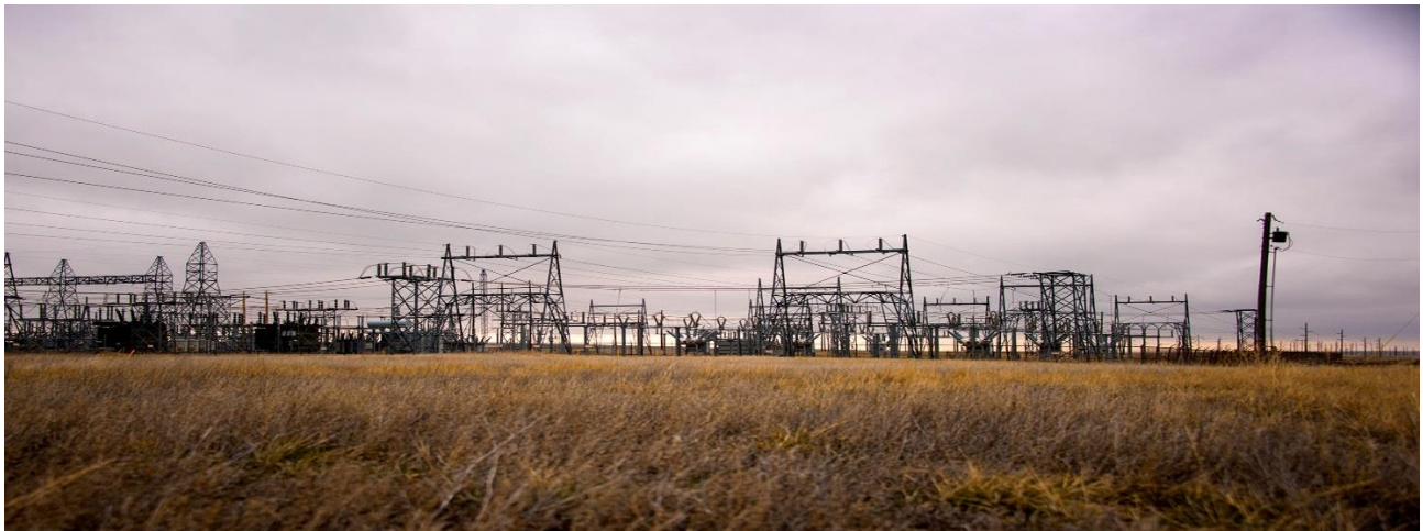
Northwestern Energy Crooked Falls Switchyard
